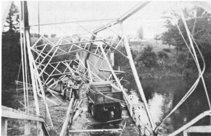
BRIDGE NORTHWEST OF LYLE — That collapsed with Osmundson Bros. truck.
